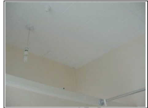
Polystyrene ceiling tiles
