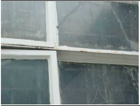
Window not shutting
