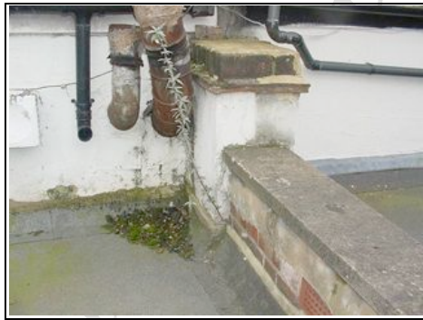
Junction of toilet roof and roof over the shop. Water is discharging onto render which is part of the reason causing dampness below
