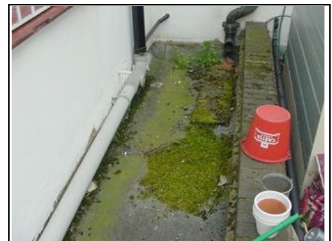
Close up of rear flat roof over the shop with moss and signs of leak below
