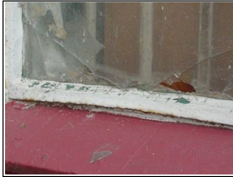
Broken glass in toilet window
