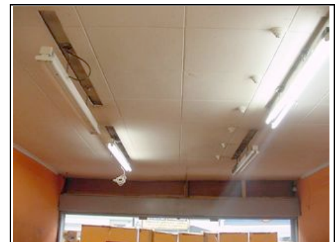
Ceiling is water damaged 15
